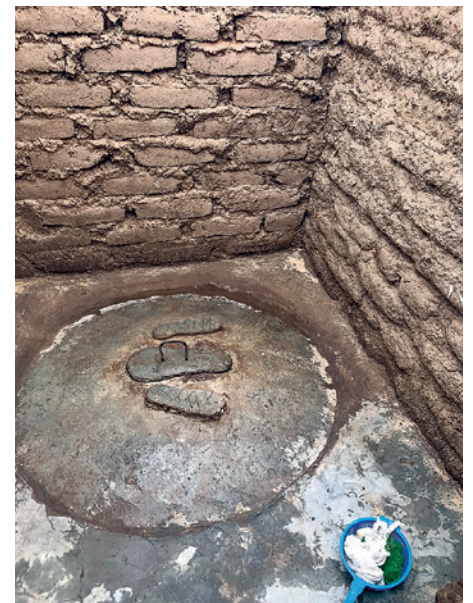
Soap for hand washing sits beside a completed latrine in a household compound in Niger. Community members dig the latrine pit and collect additional sand before the platform is installed.
