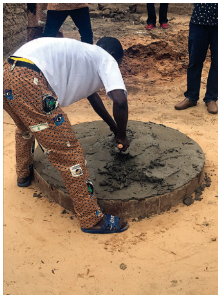
One of the more than 3,700 trained masons in Niger constructs the concrete sanitary platform that will be part of a household latrine in the community.
